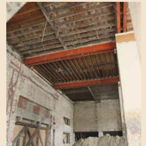
In 1953, a false ceiling was installed in a rather careless way, damaging much of the stucco.
